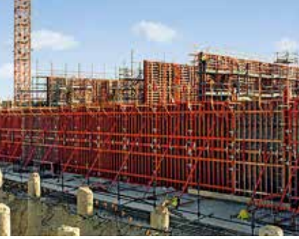
Kurnell Desalination Plant, Sydney, Australia
